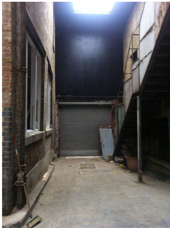
Internal elevation of Building facing Peck's Yard. This photograph shows (following installation and painting) the layer of 12mm plywood installed behind the rockwool insulation. This is the currently final internal finish of the boundary facing Peck's Yard
