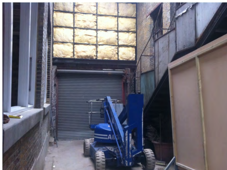
Internal elevation of Building facing Peck's Yard taken from the Atrium looking towards Peck's Yard. This photograph shows (during installation) the first 100mm layer of rockwool installed immediately behind the profiled metal sheeting.
